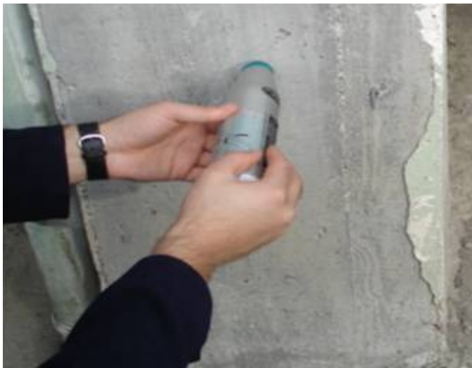
Figure 2. Schmidt Hammer test before the execution of the cores in an existing building.
