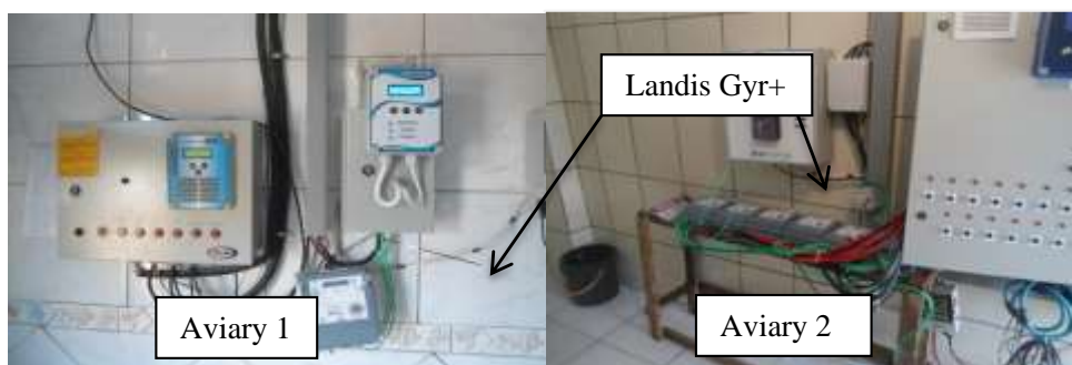
Figure 4. Measuring instruments installed in the scenarios 1 and 2.
