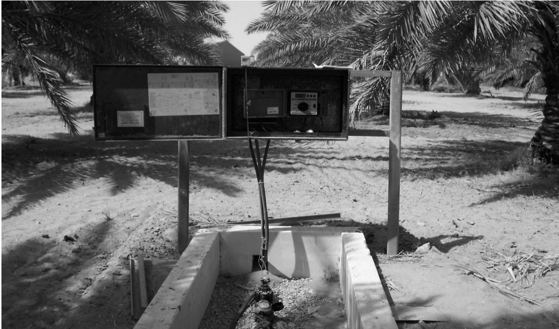
Figure 2. Total central control panel.
