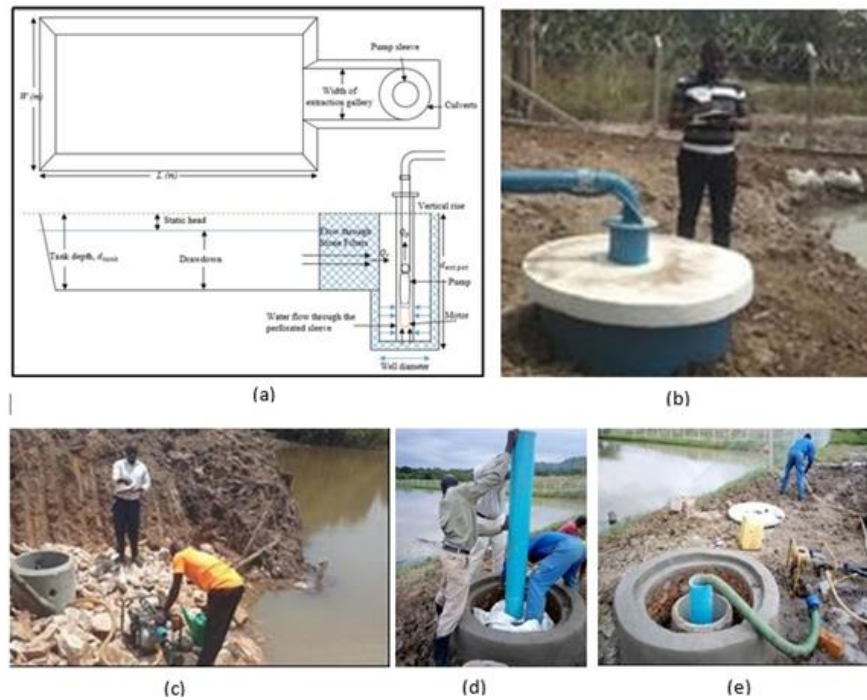
Figure 3. Modified water abstraction pot for sustainable use of submersible pump. Source: Author
