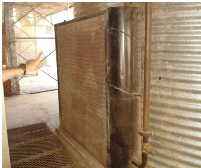
Figure 2. Heat exchanger. Source: Picture taken by the authors (2013).
