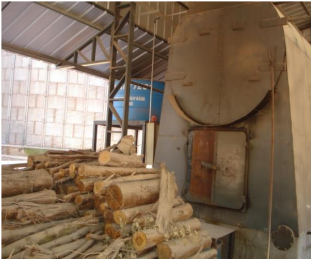
Figure 1. AWD 40 water-tube boiler. Source: Picture taken by the authors (2013).
