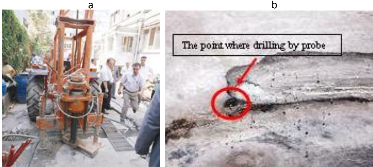
Figure 1. (a) Private real estate where drilling was done (URL-4, 2006). (b) The hole made in subway tunnel from the drilling (URL-5, 2006).
