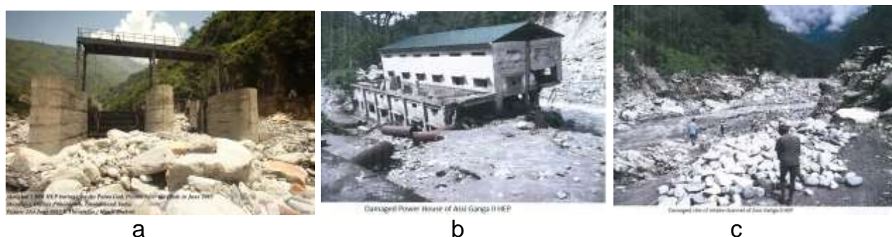
Figure 28. (a) A 2013 flood destruction of a small-size 5 MW hydroelectric project on the Piana Gad ( http://sandrp.files.wordpress.com/2013/07/e_theophilus_img_28782_lbl_rsz5mwmotighatheppithorgarh.jpg , with permission) (Picture on June 23, 2013 by E. Theophilus/Himal Prakriti); (b) The damaged Assi Ganga –II HEP power house; (c) The damaged intake side ( https://sandrp.wordpress.com/2014/06/16/uttarakhand-flood-disaster-of-june-2013-lest-we-forget-the-experience-and-its-lessons/ ).
