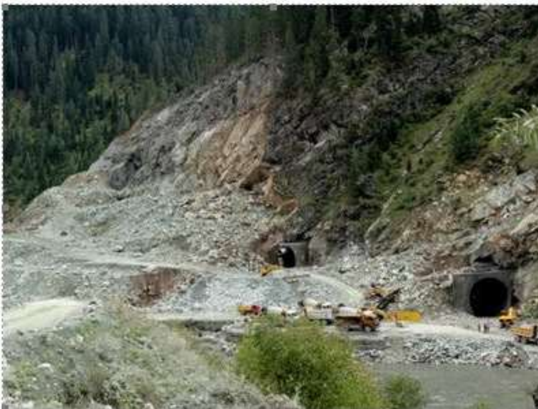
Figure 44. Tunneling at the 330-MW Kishenganga hydroelectric project in the Gurej area of Jammu and Kashmir (Photo credit: Panaromia.com, reproduced with permission from SANDRP, https://sandrp.wordpress.com/page/23/ ).
