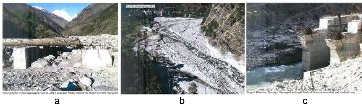
Figure 30. (a) The condition of the Madhy Maheshwar Project ( https://sandrp.wordpress.com/2014/06/16/uttarakhand-flood-disaster-of-june-2013-lest-we-forget-the-experience-and-its-lessons/ ); (b) Phata Byung HEP (76 MW, Mandakini river, Rudra Prayag district) ( https://sandrp.wordpress.com/2014/06/16/uttarakhand-flood-disaster-of-june-2013-lest-we-forget-the-experience-and-its-lessons/ ); (c) Singoli Bhatwari HEP (99 MW, Mandakini river, Rudra Prayag district) ( https://sandrp.wordpress.com/2014/06/16/uttarakhand-flood-disaster-of-june-2013-lest-we-forget-the-experience-and-its-lessons/ ).
