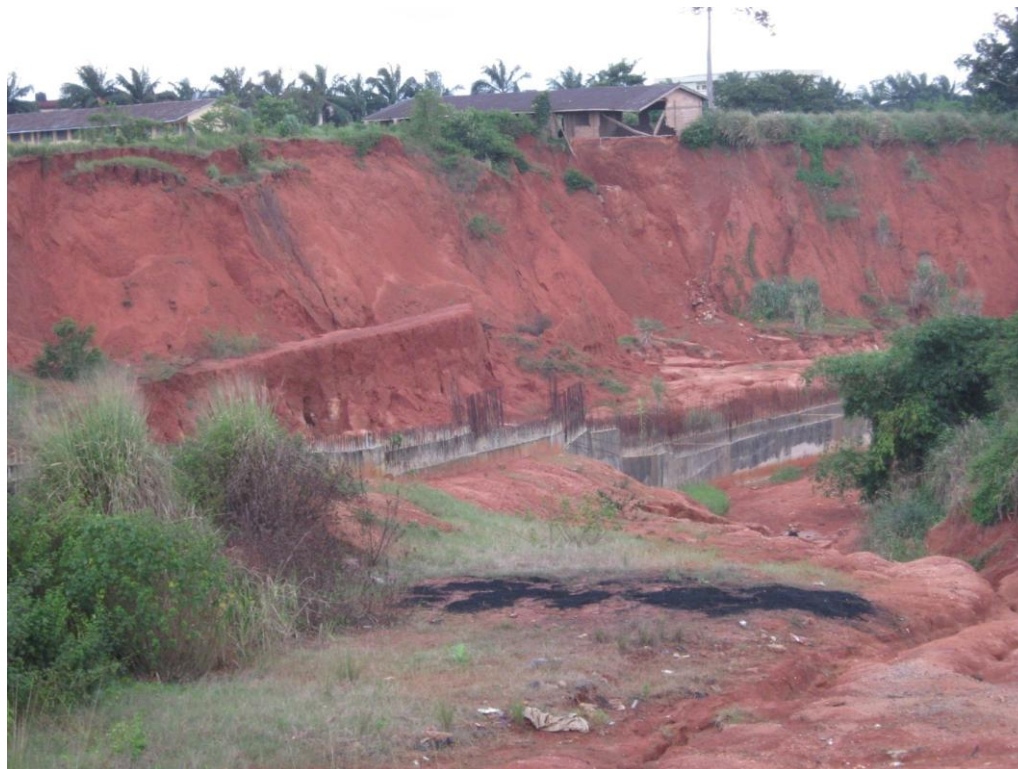
Plate 1. Ogbesan Gully, Benin City showing school building caving in and the failed community effort of drain construction to solve the gully problem.
