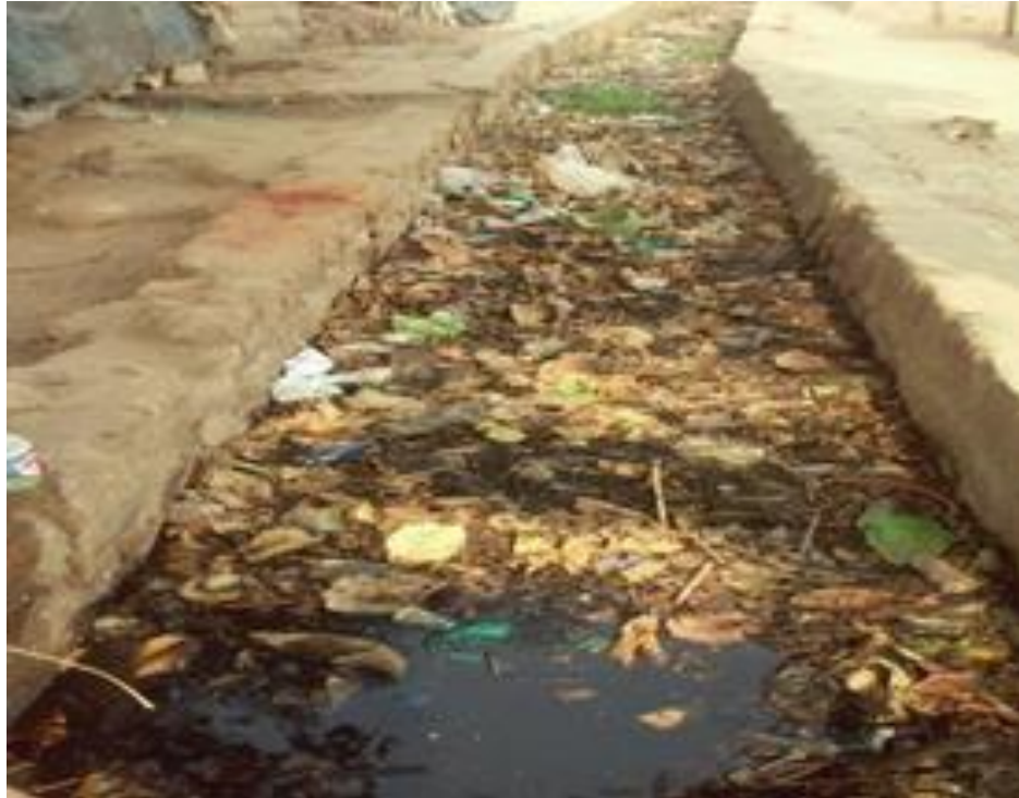
Figure 1. Obstruction of water channel by solid and liquids waste.
