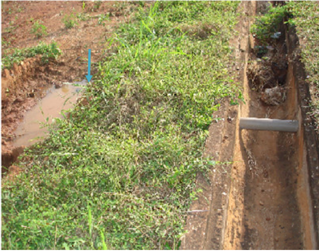
Figure 1. A broken pipe from construction work (Noguchi Memorial Institute for Medical Research, Legon, Accra, 2006). Arrow indicates direction of leakage on pipe.
