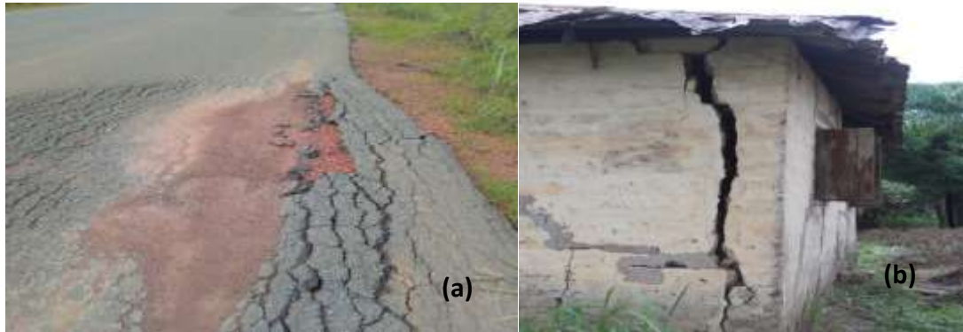
Figure 1. Evidence of failure of engineering projects in the studied area.
