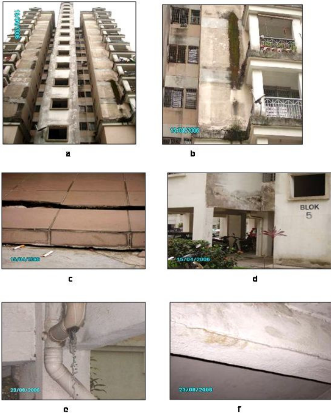
Figure 3. Façade and services defects at post occupational stage.
