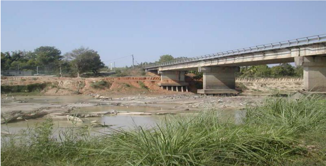
Figure 1. Bridge pile exposure due to sand extraction at Jambatan Baru Kuala Ketil (Ab Ghani et al., 2003, quoted by Abdullah, 2002).
