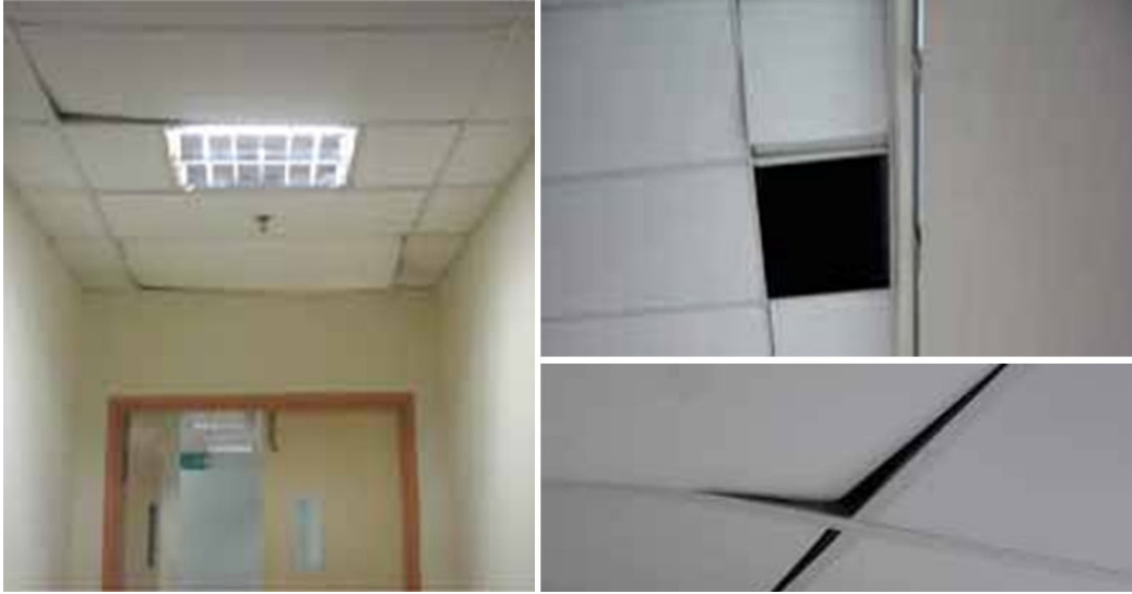
Figure 1. The broken ceilings in LESTARI.
