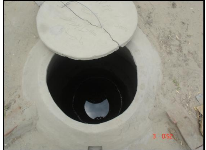
Figure 4. External structure of a cistern or storage tank found in the Nangarparkar region of Thar Desert of Pakistan [Photo credit to the first author].
