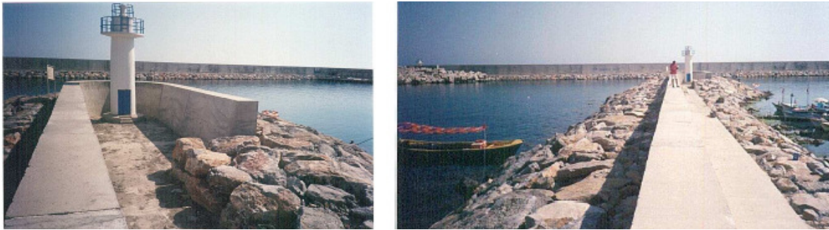
Figure 2. General view of the marina and breakwater built by using natural stones (schist and limestone) in the inner harbor (lighthouse region).
