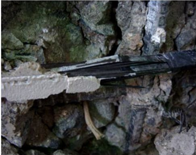
Figure 6. Damage of CFRP strip after testing.
