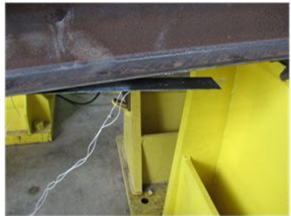
Figure 8. End debonding (EDB).
