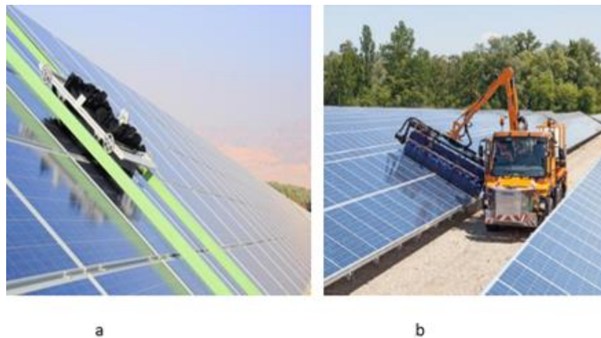
Figure 2. (a) Waterless cleaning of solar panels via robot and b) FWG panel washer.
