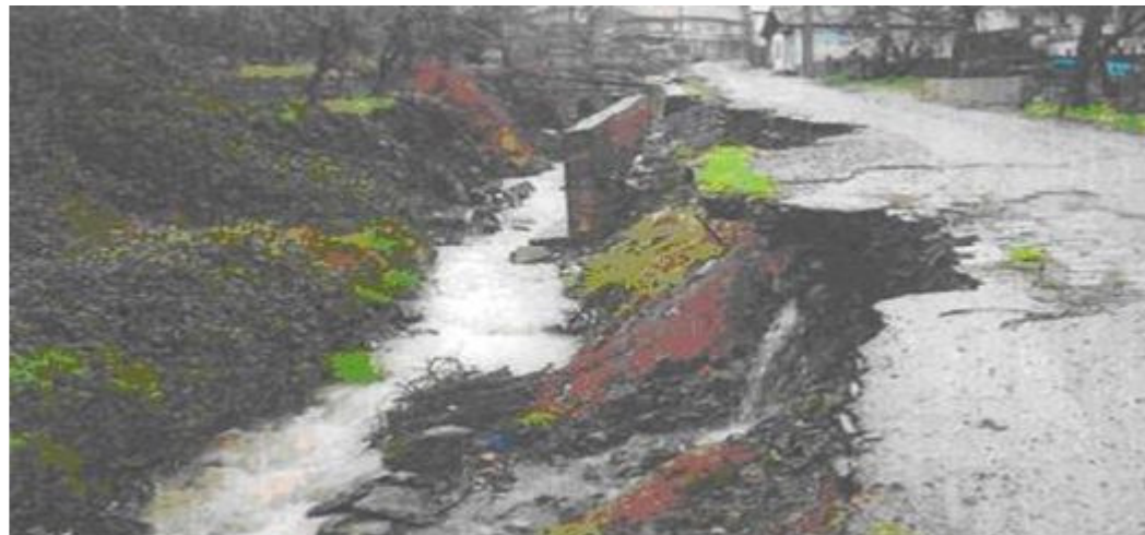
Figure 6. Damage to the wall along Kilic Stream (DSI, 2007).
