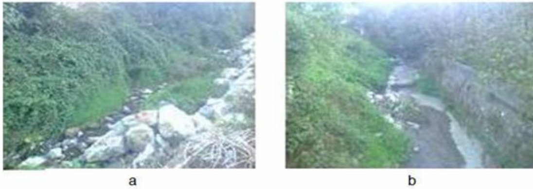
Figure 14. a. The unsupported slopes of b. The rehabilitation dike across Kilic Stream.
