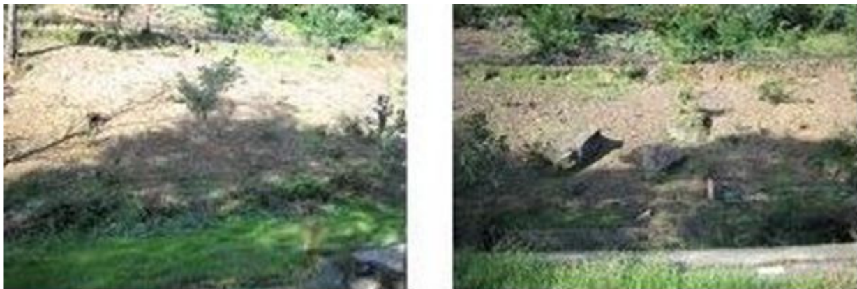
Figure 15. The sections of the slopes of Kozlu Stream where the vegetation cover has decreased.
