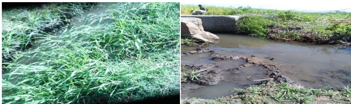
Figure 4. Canals covered by weeds and mud.
