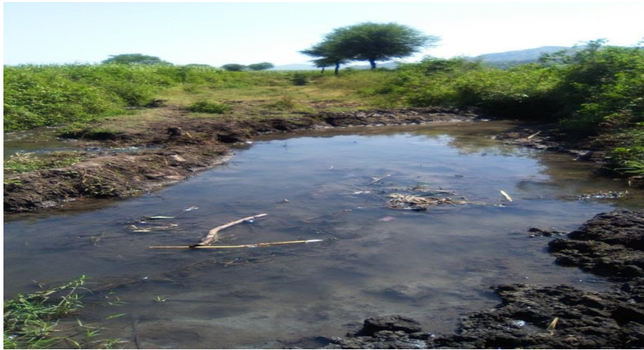
Figure 5. Silt deposition in tertiary canal.
