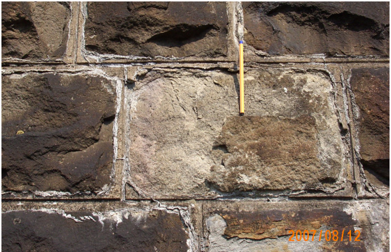
Figure 5. Stone surface damage by single scales and fragmentation into sand-grain size, intense linear salt efflorescence at stone's margins, blackening stone surface.
