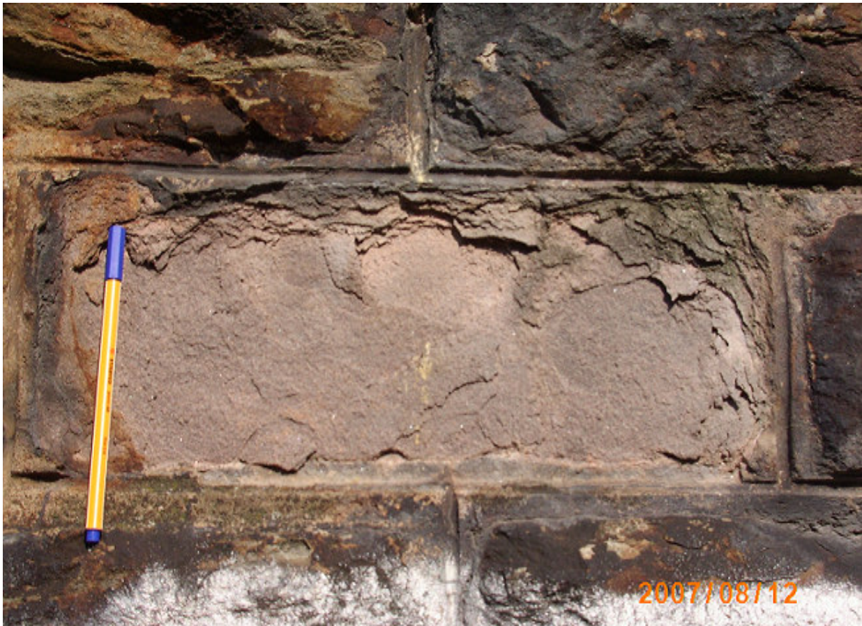
Figure 3. Back weathering and multiple scaling, white salt efflorescence and blackening of stone surface of construction rock of the walls under investigation.
