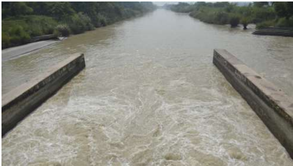
Figure 8b. Cleaning of Upper Ganges Canal ( http://www.hindustantimes.com/noida/cleaning-of-upper-ganga-canal-begins-no-water-supply-till-oct-21-jal-nigam/story-R3MFqtlr3nNwHJeEpwh43J.html ; (Photo by Sakib Ali /Hindustan Times).
