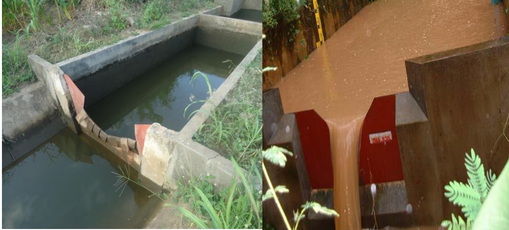
Figure 10. Condition of the main canal in blocks with lowest conveyance efficiency.
