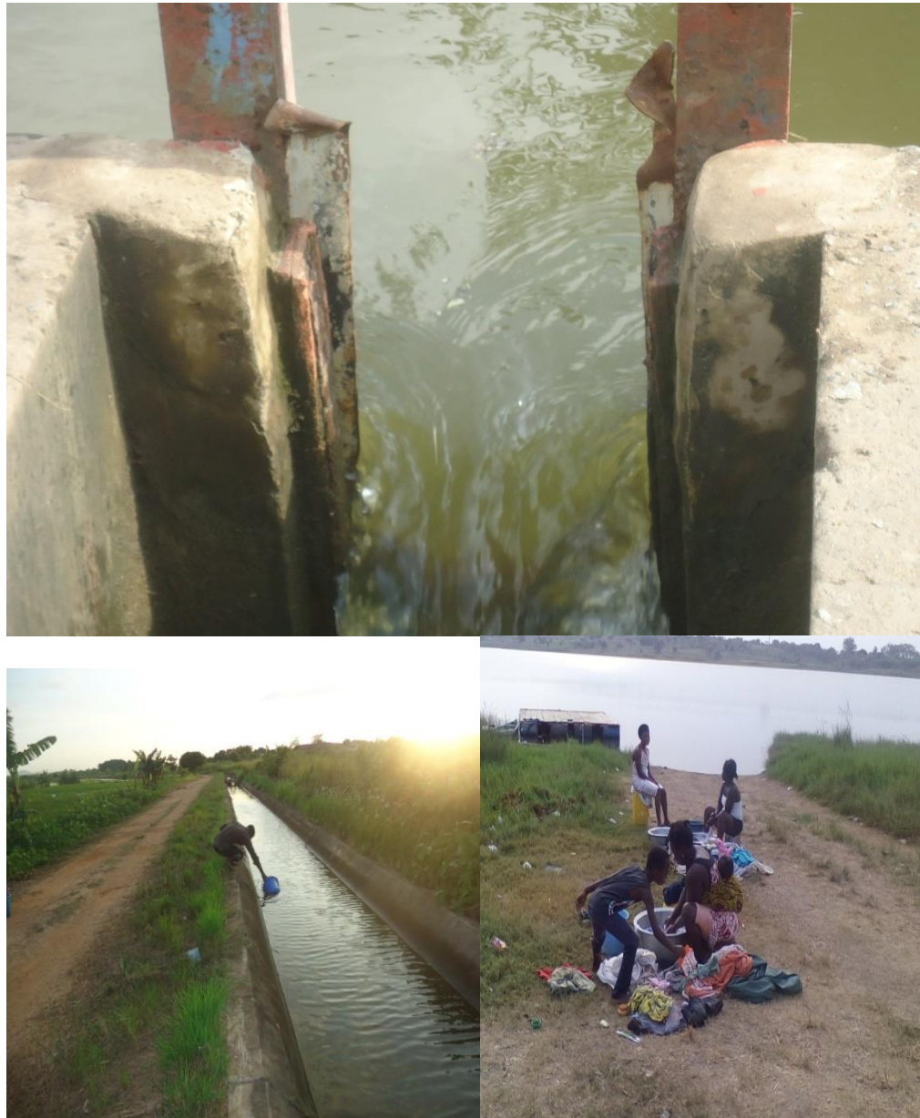
Figure 9. Broken check gate and Water used for domestic purposes.
