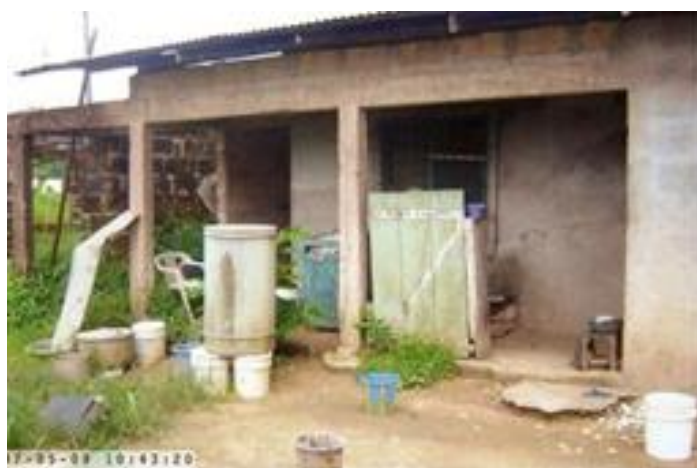
Figure 14. Chief Benjamin's one-story building at Okoroba village with a temporary roof covering over a part of it.
