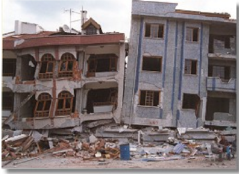
Figure 1. Building pounding (New Zealand, 2009).
