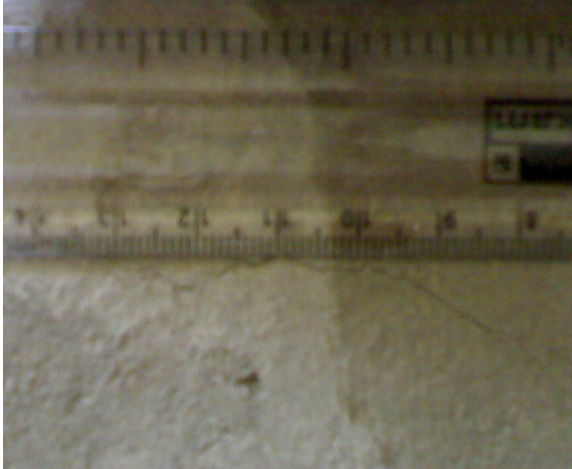
Figure 2. Shrinkage crack of Mix 1.
