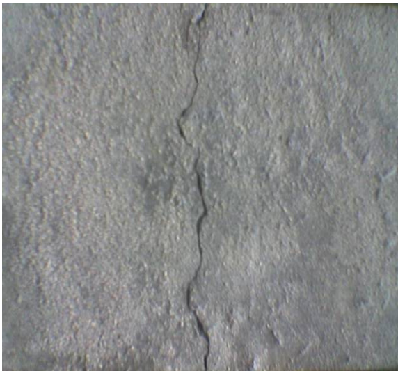
Figure 3. Shrinkage crack of Mix 2.
