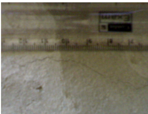
Figure 4. Shrinkage crack of Mix 3.
