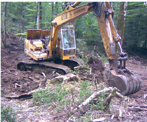
Figure 2. Clearing and grubbing by hydraulic excavator in Agha Mashhad forest of Hyrcanian zone.
