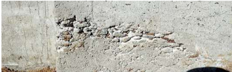
Figure 13. Honeycombs on concrete.
