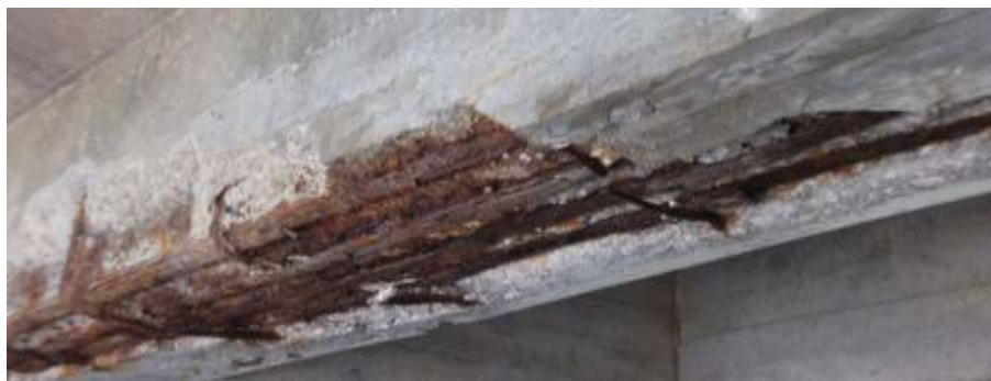
Figure 9. Corrosion of reinforcement. Source: Adapted from concreteprotection.com.
