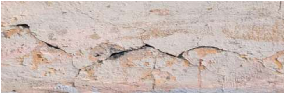
Figure 11. Spalling of concrete. Source: Adapted from https://cp-tech.co.uk/news/causes-effects-and-repair-of-concrete-spalling .
