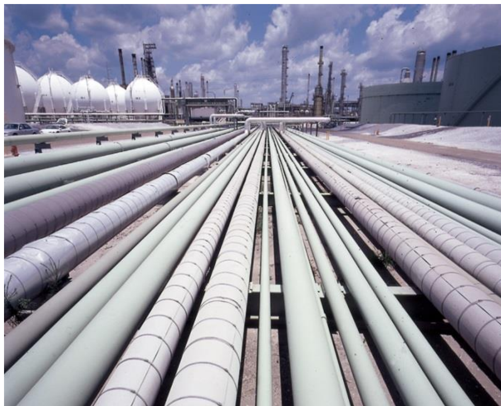
Figure 16. Above ground oil pipelines.
