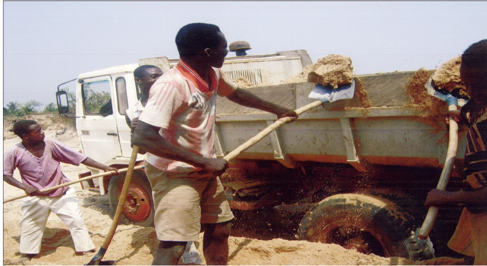
Figure 2. Young men manually loading of a truck in a quarry using shovels.
