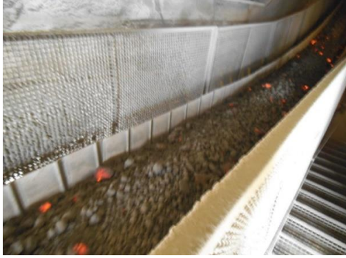
Figure 1. Pan conveyor carrying red-clinker. Source: (Oyepata et al., 2020; Oyepata et al., 2021)
