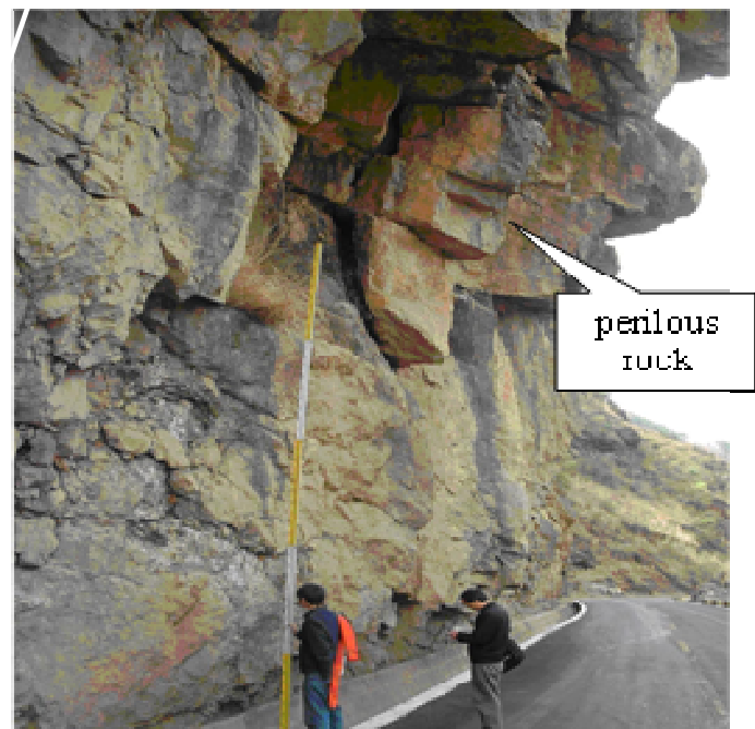
Figure 6. A falling perilous rock.
