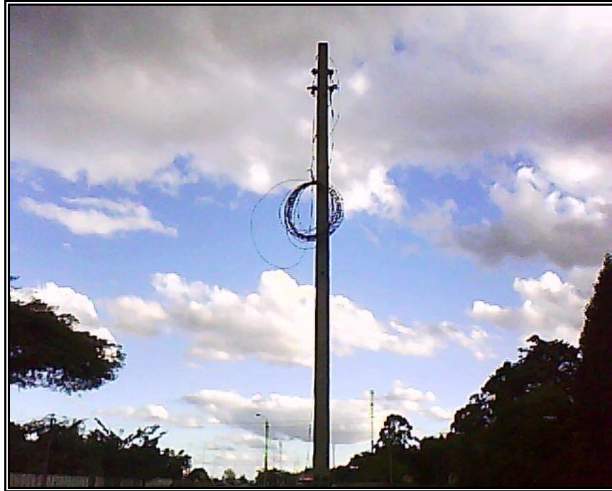
Plate 3. Typical broken wiring in Marlborough East.
