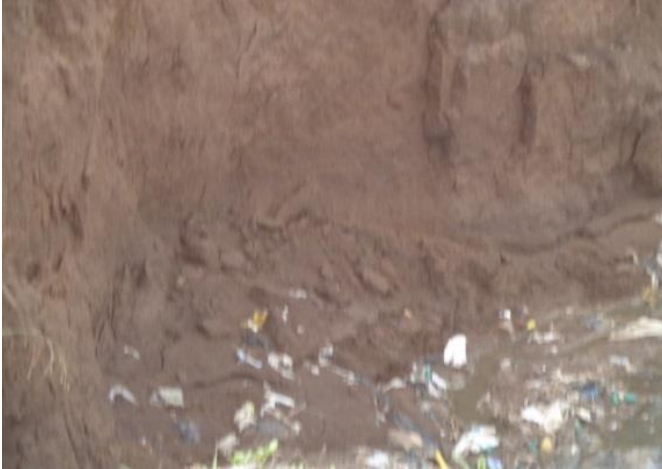
Figure 8. Collapsed outer bank. Monene, 2014: Photographs were taken 10 m downstream of Kangundo Road Bridge on 17/12/2013.
