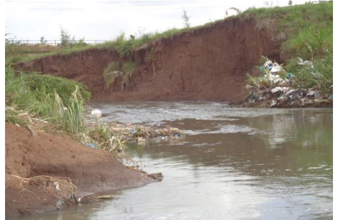
Figure 5. Land slide of high river cliffs. Source: Monene, 2014: Pictures taken on 17/12/13 and 5/9/13.
