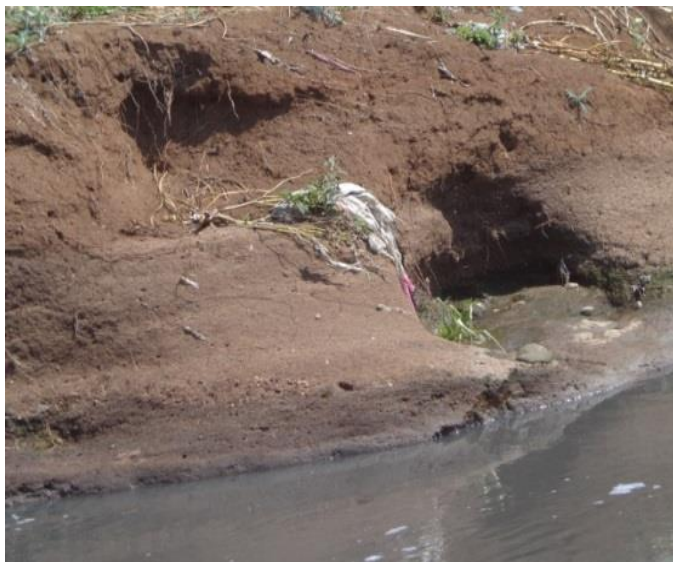
Figure 12. Pop out failure results to cavities. Source: Monene 2014: Photos taken on 17/12/2013 during wet season) and 5/9/2013 during dry season.
