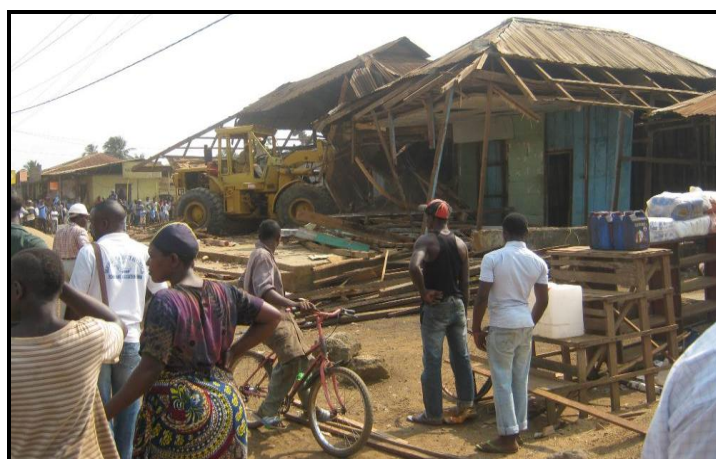
Figure 4. The demolition exercise in Fiango-Kumba (notice a caterpillar on duty as the population watch in anguish).
