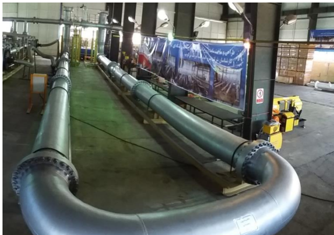
Figure 9. Bidirectional prover of Genaveh 10 Million BBL crude oil storage tanks fiscal metering system project – Designed and fabricated by Asia Instruments Co. LTD.
