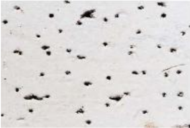
Figure 5. BioBlock Plus ceiling panel signifying no visible mold growth.
