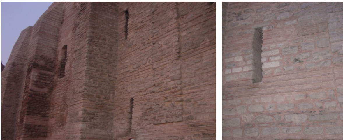
Figure 8. The photos of the repair mortar after one year, during the restoration of Anemas Dungeons.
