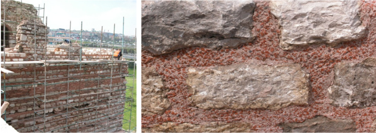
Figure 7. The photos of the repair mortar used during the restoration of Anemas Dungeons (2006).
