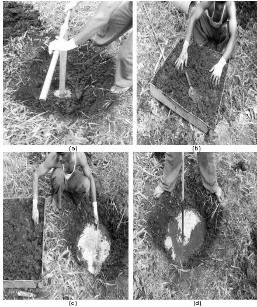
Plate 1. Installation of column. (a) Drilling augur, (b) Mixing soil and binder, (c) Insert mixed soil and binder, (d) Tamping by steel rod.
