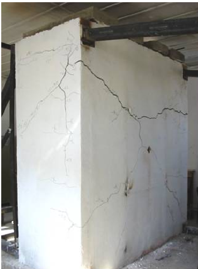
Figure 4. The cracking pattern of Wall A at ultimate stage.
