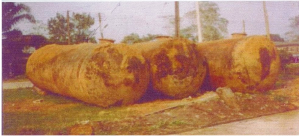
Figure 1. A typical petrol storage tanks from Uniport filing station. (Installed In 1977 and Failed in 1996).
