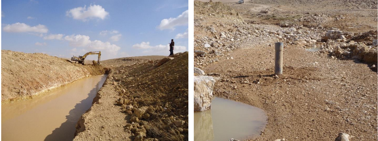
Figure 10. Left side: excavation of the 90 m long trench along the old wadi channel. Right side: the restored wadi section: below the front part is the now covered groundwater dam, behind the observation and pumping well and in the background the refilled wadi section used as groundwater reservoir. The picture shows the rebuilt wadi section after the first flood event.
