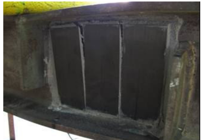
Figure 9b. Procedures of CFRP failing.
