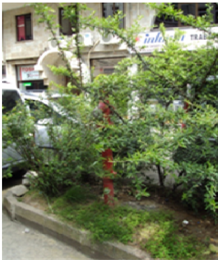
Figure 5. Example of the lack of visibility of some hydrants covered by plan.
