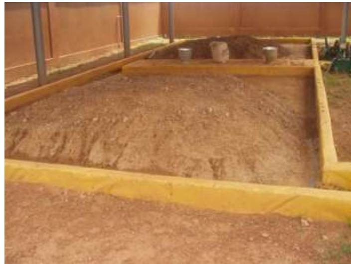
Figure 2. Processing platform for the pilot sample of polluted soil and some accessories at the Ouaga III station of SONABEL.
